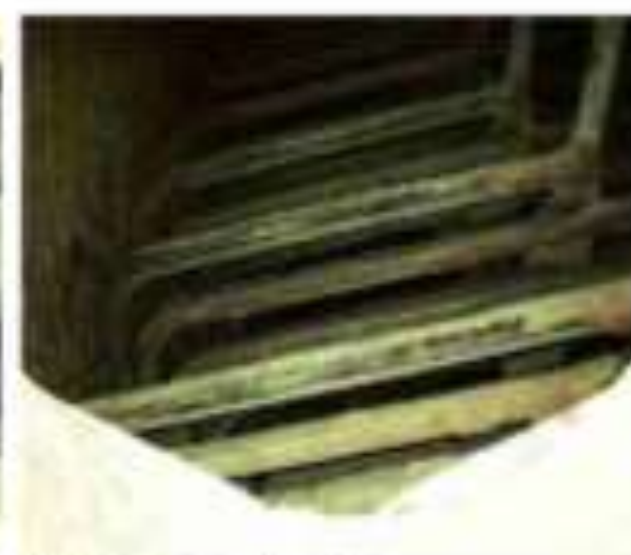
After an on-line cleaning
