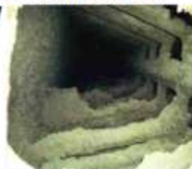
Before an on-line cleaning
